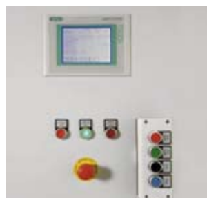
Siemens control system
